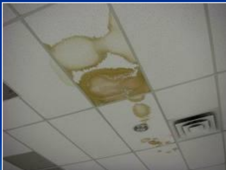
Stained ceiling tiles
