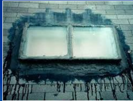
Evidence of leaks
