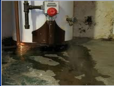
Mechanical system leaks
